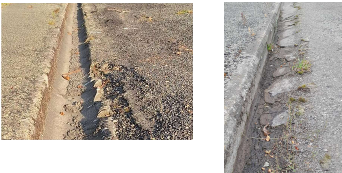
Figure 9.37 - Very Poor Condition Rated Kerb and Channel
