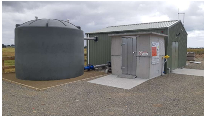
Manchester Bore Treatment Plant December 2019
