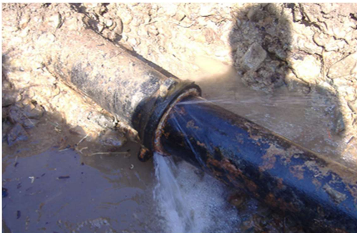
Figure 8-4: Cast Iron Pipe Failure
