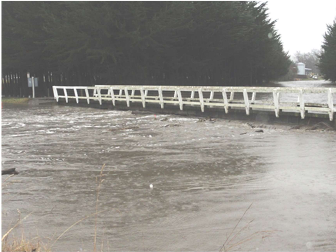
Holme Station Corner Bridge in Flood conditions
